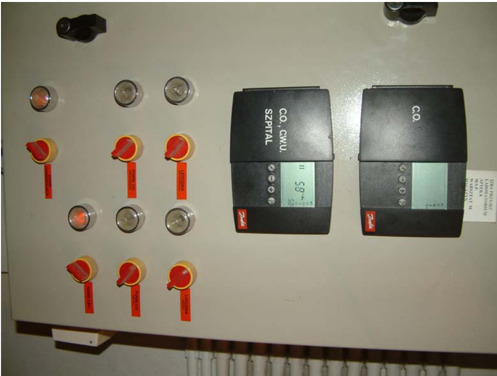
Figure 3: Controller with outdoor temperature sensor is installed in the heat centre. Controller adjusts heat factor flow dependent on outdoor temperature.
