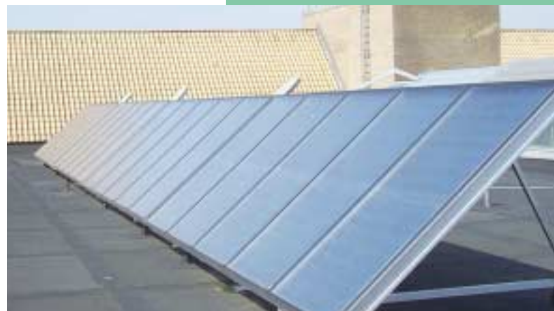
Solar Collectors at Aabenraa Hospital
